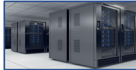
Small Control room
