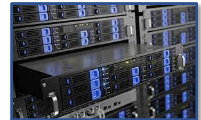
Data Center system
